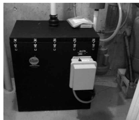
Figure 12 Installed AIRraider™ 433-S
